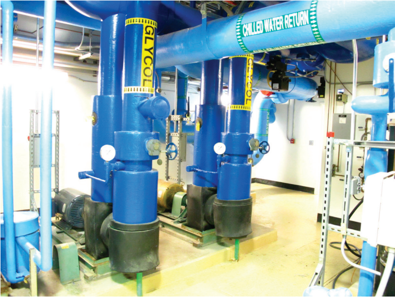
The peak cooling loads occur at the exact time of the highest peak electrical rates. This is why TES systems are so valuable; they reduce the energy consumption and demand during peak.
